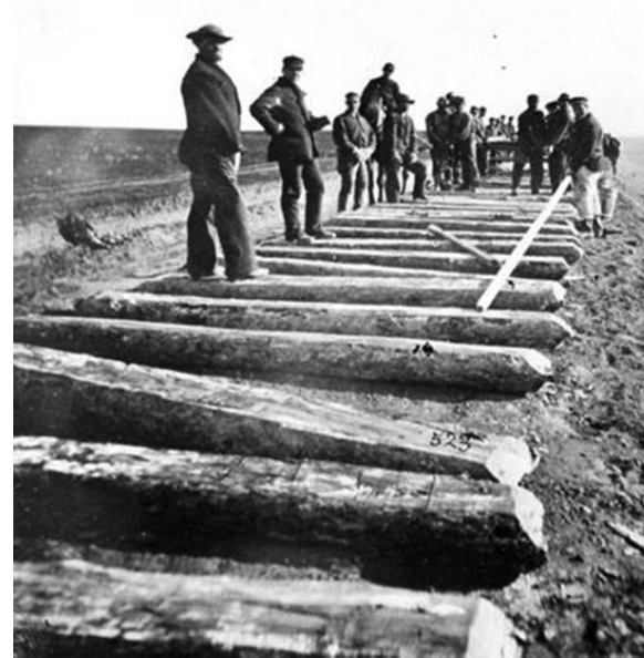
Track layers prepare roadbed and lay cross ties as the Northern Pacific approaches the Red River.
